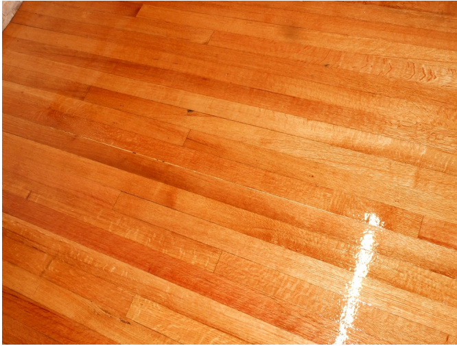
Figure 14: Because we waited more than a month (it was several) between the second and third coats, we found the wood moving due to humidity changes. This allowed for some final wood filler in some cracks that appeared. It's possible the tar paper and tiles on before would've kept the wood from moving, in the past.
